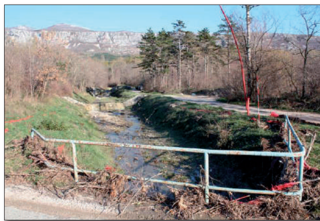
Figure 4 Riverbed section of Slani Potok where the flash flood occurred with visible water table traces.
