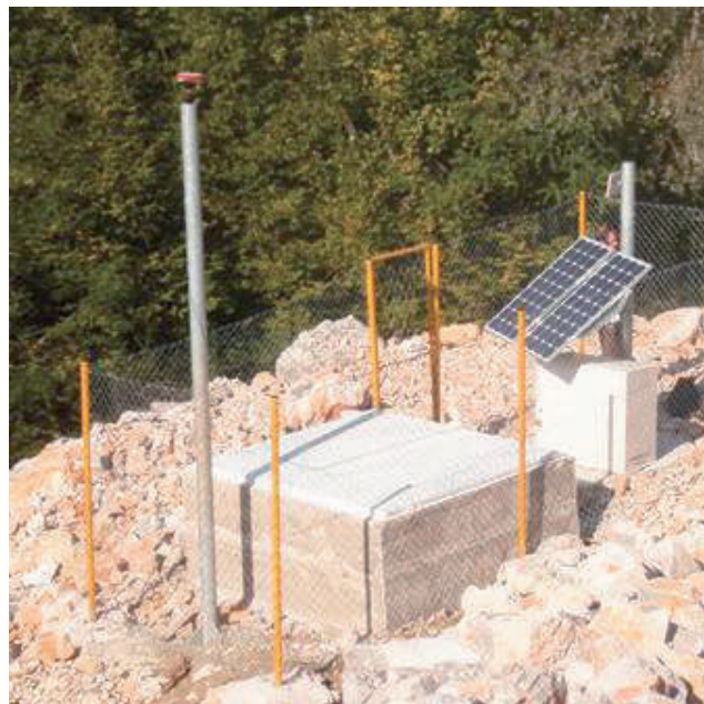
Figure 3 GPS rover and solar panel installation. Concrete box is round up construction for geotechnical monitoring equipment protection (Arbanas et al. 2012a).
