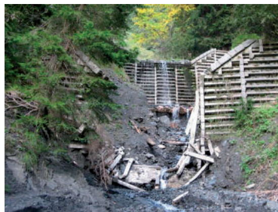
Figure 8 Example of a collapsed check dam.
