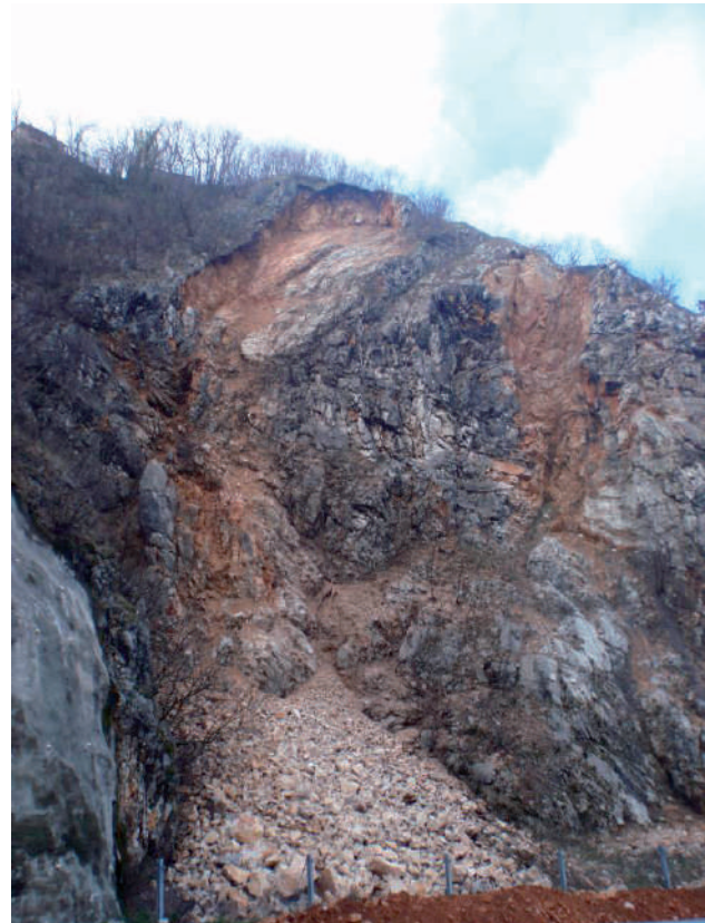
Figure 2 Rockfall of 500 m 3 occurred on the state road Rijeka-Orehovica, Banska Vrata location, March 2013.
