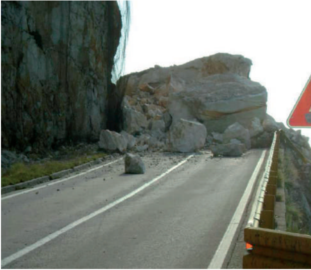
Figure 1 Rockfall of 700 m 3 occurred on the state road Makarska-Vrgorac, Stupica Location, October 2010.
