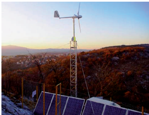
Figure 2 Mini power plant at the Veli Vrh location consisted of 1 KW 6 solar panels and 500 W windmill.
