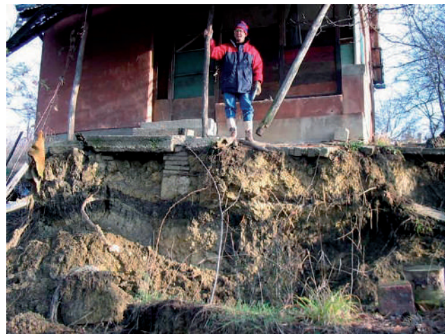
Figure 4 Deformation on the house.
