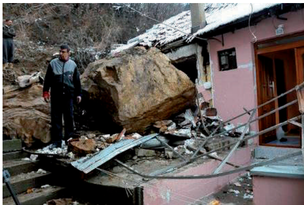
Figure 5 House in the City of Tetovo destroyed by rock fall on 9 February 2013.
