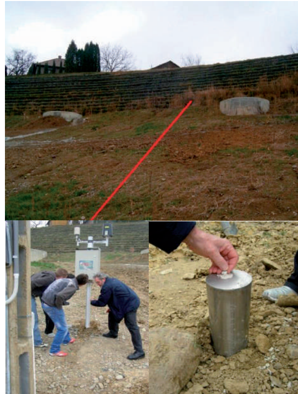
Figure 3 Monitoring alignment (red line) and installed surface sensor system and inclinometers - zone 1.
