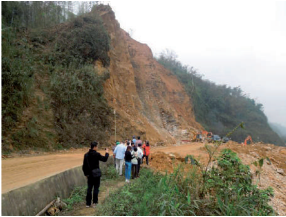
Figure 1 Landslide at the National Road No. 6, Hoa Binh Province.
