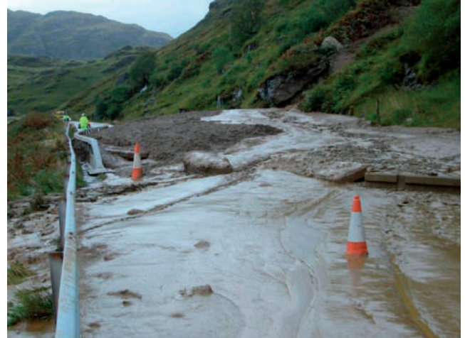
Figure 1 Debris blocking the road after event 2009 (picture source Scotland Transport).
