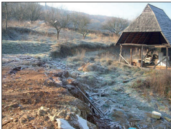
Figure 2 Cluj Ethnographic Museum house affected by landslides.
