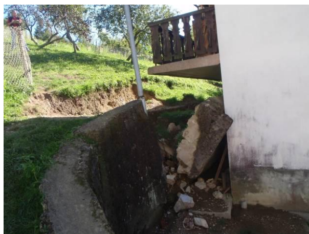
Figure 5 Example High Risk landslide.
