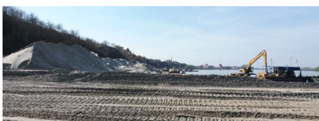
Figure 10 Construction of the planned embankment for the waste water treatment facility (UPOV) in Vukovar.
