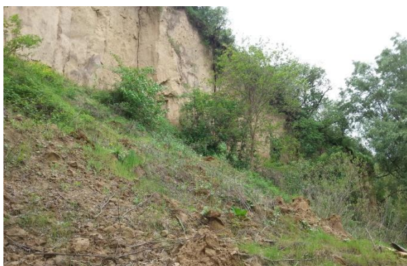
Figure 7 Tensile cracks observed along the forefront of recent instability in Vukovar.
