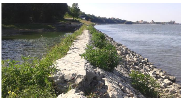
Figure 9 The crown of the stone embankment leaning back, warning of possible instability.
