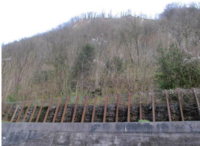
Figure 2 Steep slopes in Triassic dolomitized limestones above the road (road section between 12.500 and 13.000 km). The road is protected by a non-flexible net barrier and gabions.
