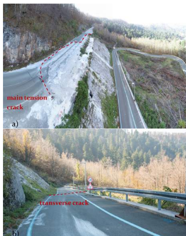
Figure 2 Evidences of the landslide movements: a) main tension crack on the state road D3, b) subsidence of the local road towards the Lokve Lake.
