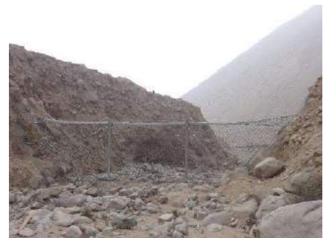
Figure 7 UX- barriers with two posts in the channel bed
