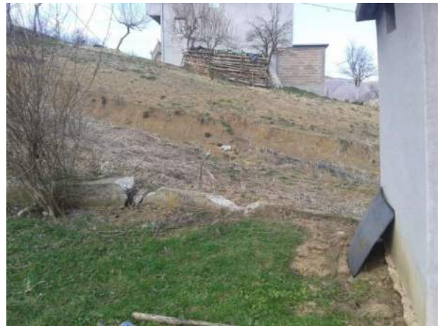
Figure 5 Dumped the retaining wall next to the house
