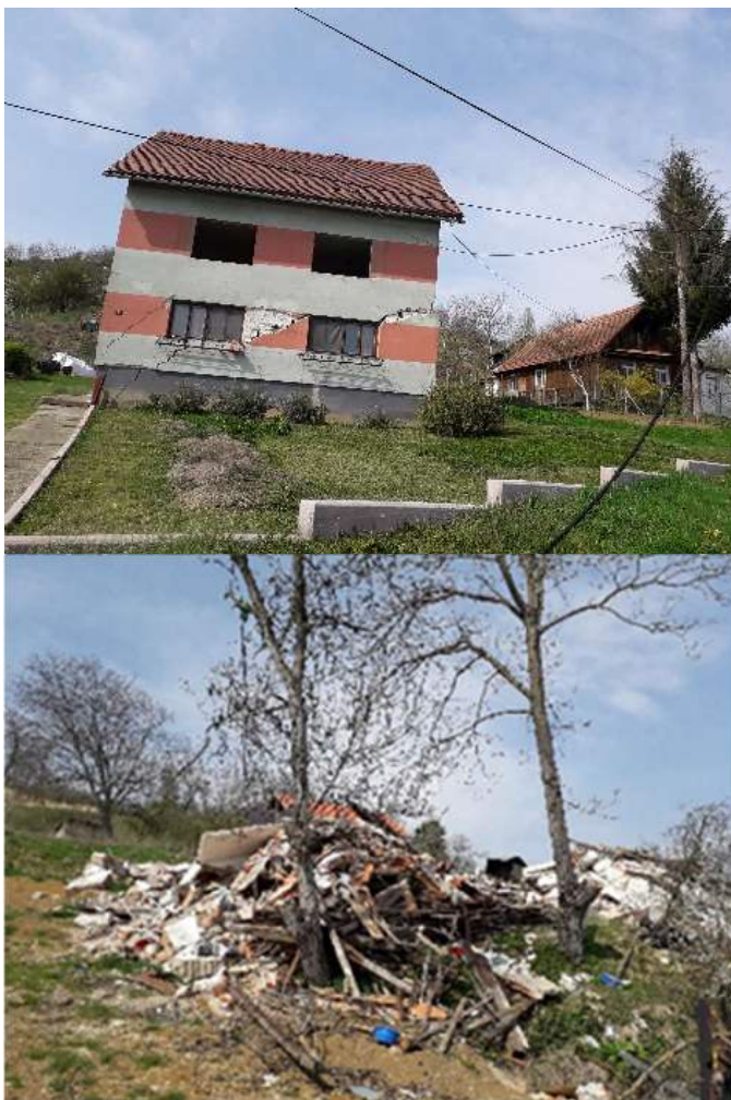
Figure 3 Houses destroyed by collapse of the Hrvatska Kostajnica landslide on 13 th March 2018.
