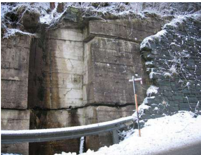
Figure 2 Damage to retaining walls along "old" route
