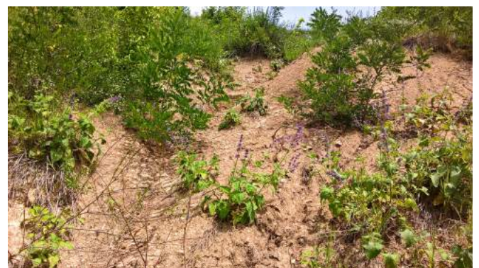
Figure 2 Sediment erosion on the slope
