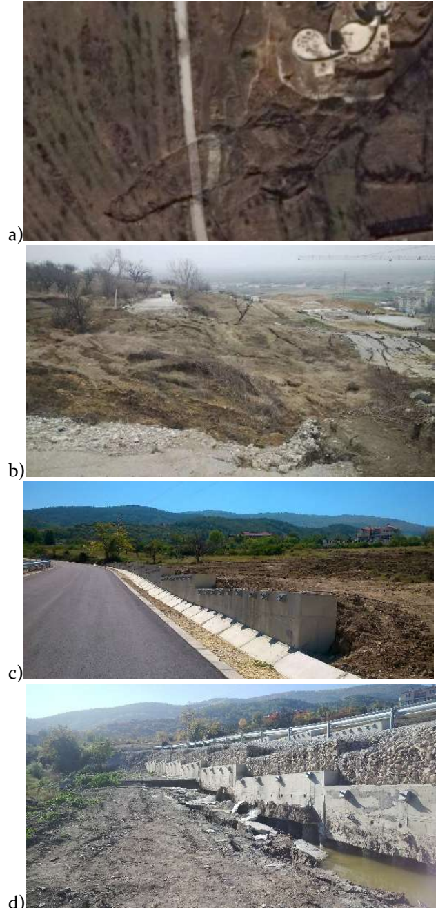
Photo 1 a) Satellite image of the landslide. b) Displacement of the road. c) Local stabilization of the road. d) Slide after the execution of the primary stabilization.
