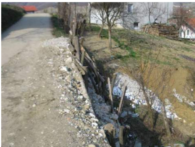
Figure 4 Damaged local road
