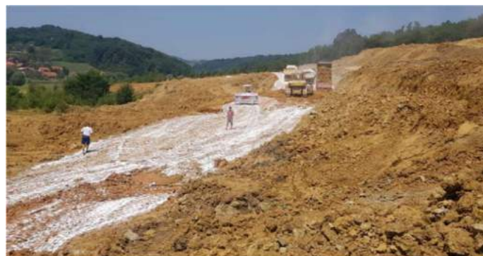
Figure 13 Construction of an embankment during clay pit remediation. A sandy layer of lime is visible, which is compacted with "hedges" before installing the next layer
