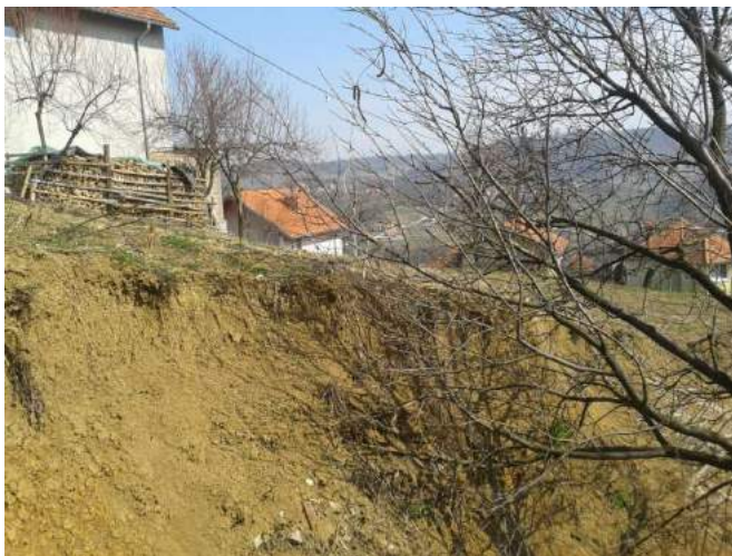
Figure 3 The landslide scar
