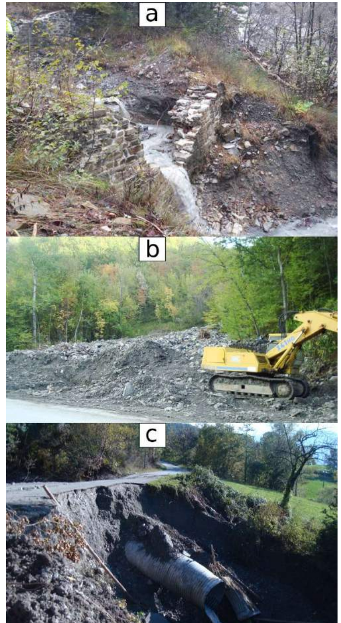
Figure 5 Example of effects on infrastructures in Parma province: a) check-dams cut-through by debris flows; b) road overrun by debris; c) erosion and cut-through of the road track.
