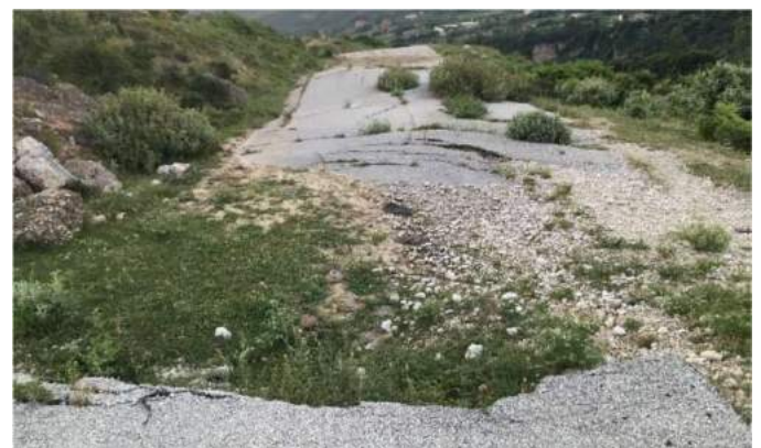
Figure 2 Landslide view, km 7+500[2]
