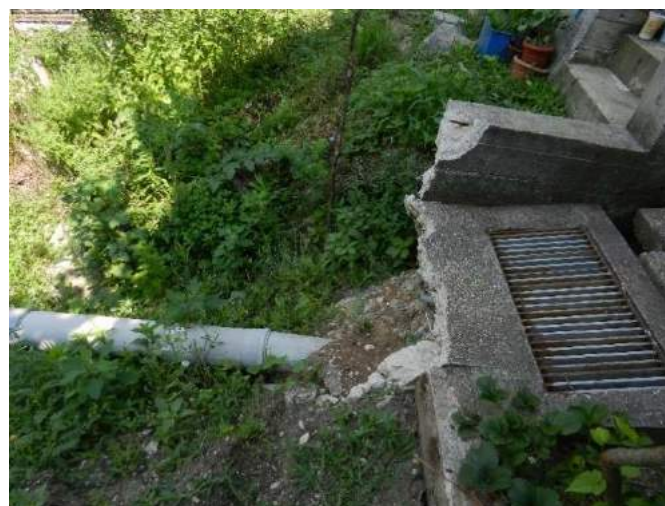
Figure 6 Fracture of the concrete wall below the house (Nikolic T. 2018)
