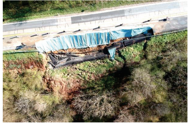
Figure 3 Aerial view of Dubravci landslide on the state road DC3 (section 015) at km 2+060.
