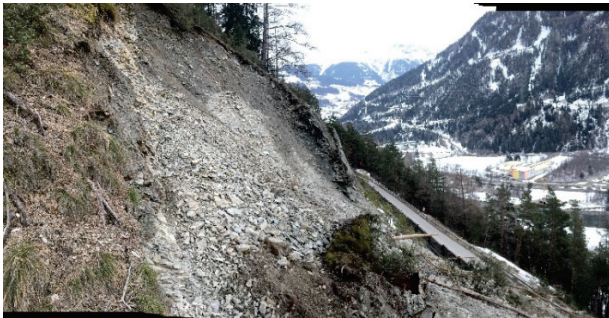
Figure 5 View from the top of the landslide along the Ladiserstrasse.
