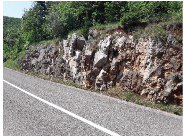
Figure 3 Example of the slope with three discontinuity sets plus random discontinuities (segment from km 16+530 to km 16+640)
