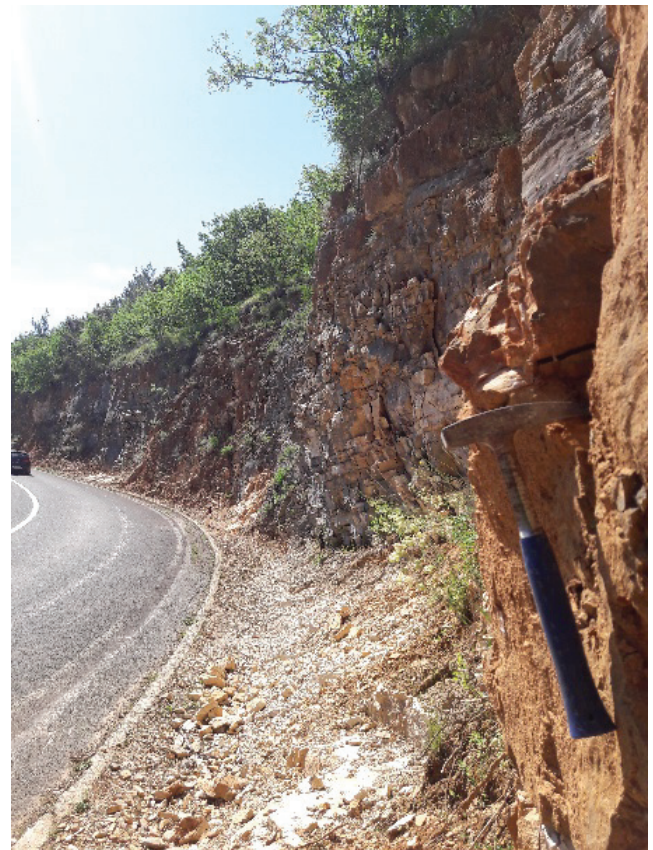
Figure 2 Example of the slope with a high degree of undercutting (segment from km 18+950 to km 19+150)
