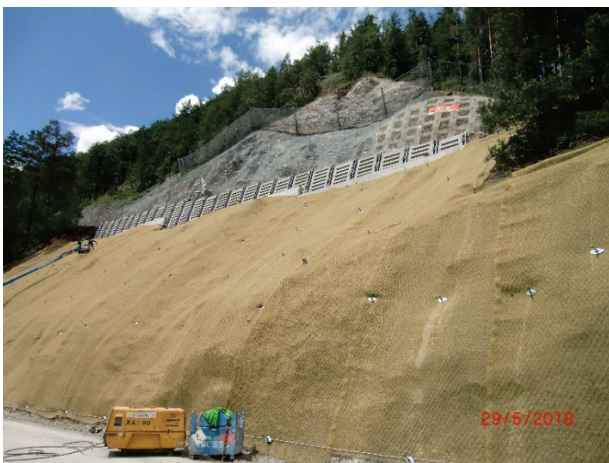
Figure 15 Final works underway at the Serfauterstrasse, with a highlight on the greening mat along the bottom part of the road.
