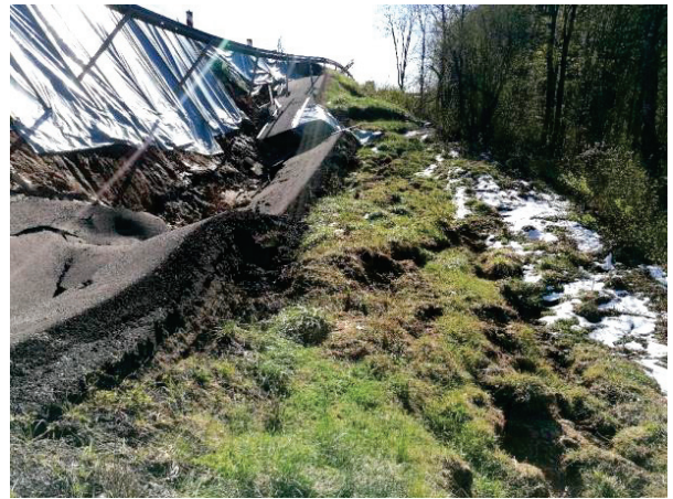
Figure 4 Main scarp of the Dubravci landslide.
