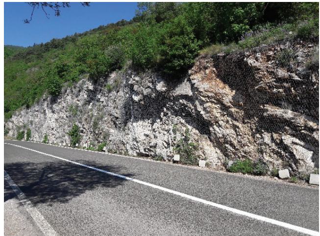
Figure 1 Example of the slope with major launching features present (segment from km 19+300 to km 19+490)
