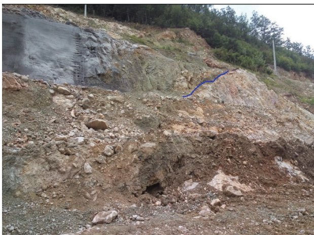
Figure 4 Left boundary of an active landslide.
