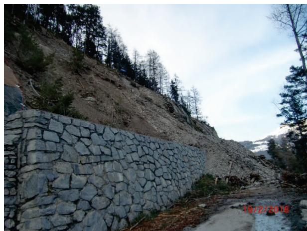
Figure 4 View from the blocked Ladiserstrasse, where a large part of the slope failed after the extreme weather conditions in January 2018.
