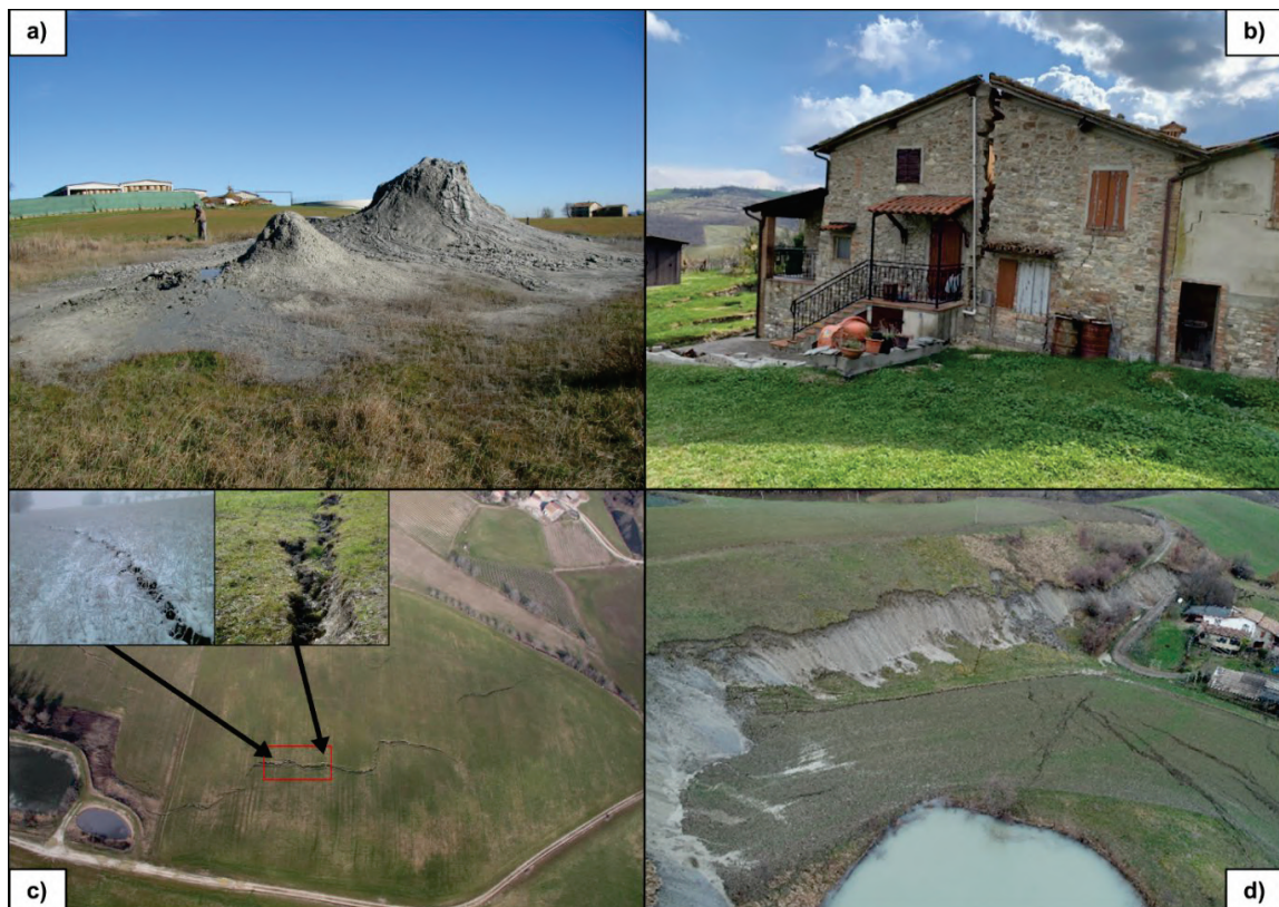
Figure 1 Field impressions of Madonna di Puianello field calderas. a) Active mud volcanoes in the Possessione field; b) Houses damaged within the Traino caldera; c) and d) normal rimming fractures in the Possessione and Traino fields. Picture (c) courtesy of G. Bertollini.
