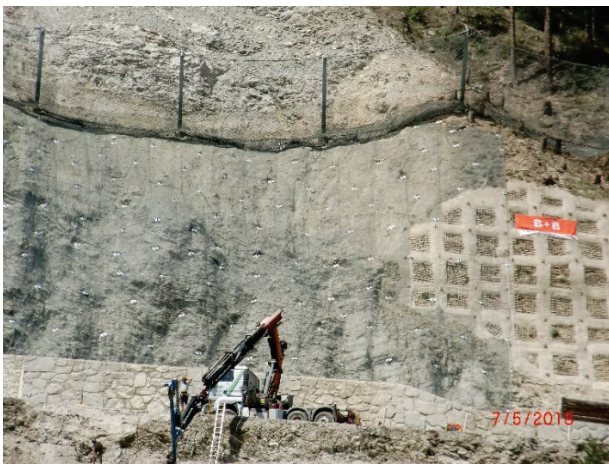
Figure 14 Drilling truck starting on the stabilisation works at the bottom part of the Serfauterstrasse instability.
